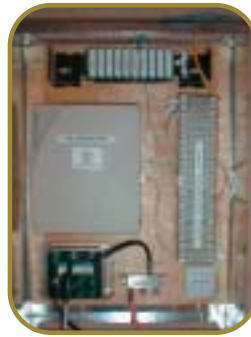
Home Control Center in the garage contains phone and video patch panels and hub/router which serves as a gateway and firewall.
